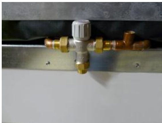
DHW heat exchanger installed
